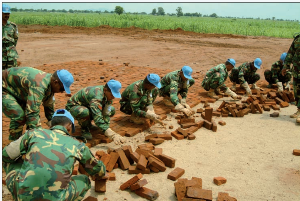
Peacekeepers from Bangladesh busy with road construction work in Juba, Sudan, 18 July 2005.
